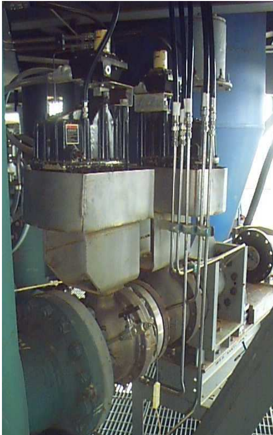
Close-up view of isolation valves with nitrogen purge and vent lines
